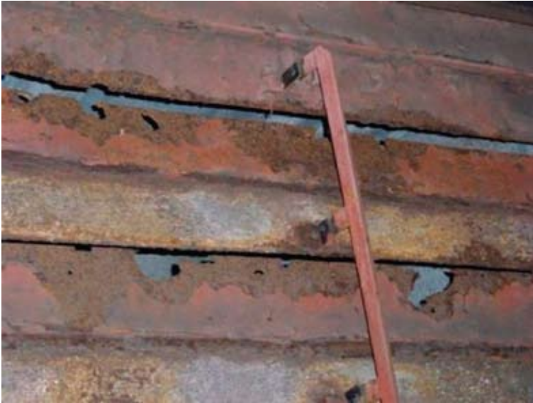
Engine room fire damper louvers corroded
