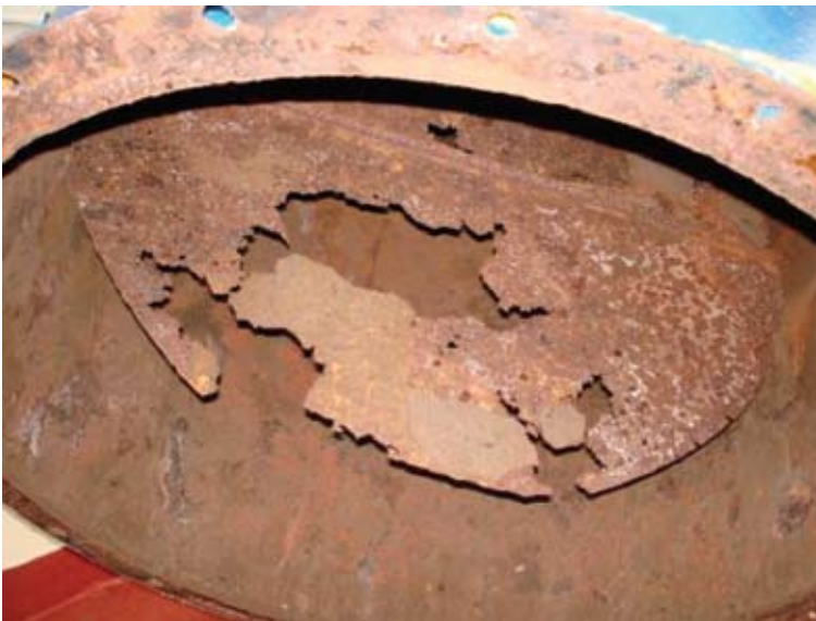
Engine room fire damper
