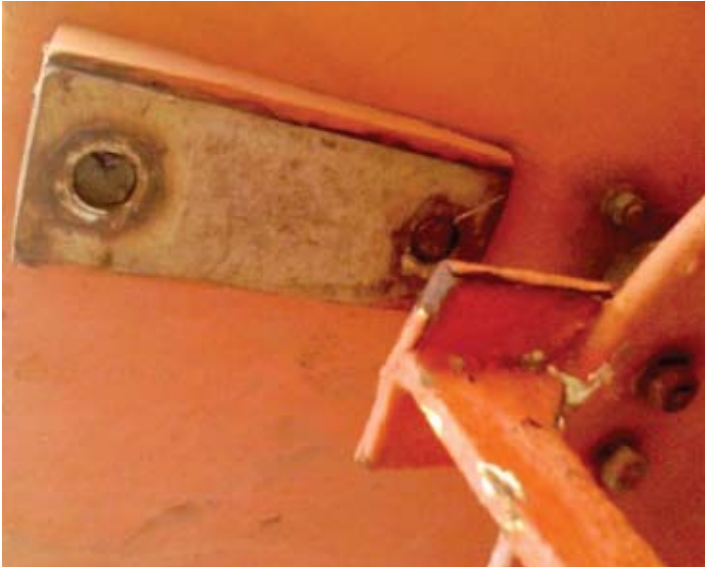
Lifeboat hook securing arrangement - bolt heads sheared off
