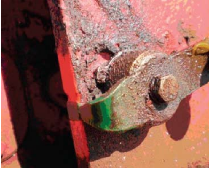
Lifeboat release hook incorrectly reset - indicating groove no longer the reference for fully locked position
