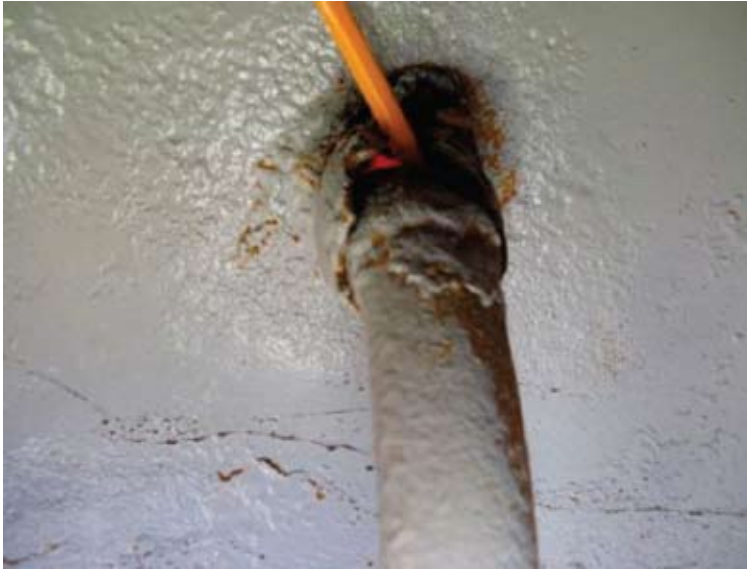
Cargo hold CO2 line holed
