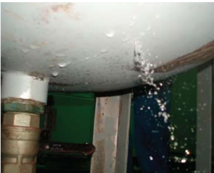
Oily Water Separator main body leaking
